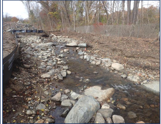
(right) Same area as the photo above but taken from the opposite side. Large rock weirs (like one in bottom of photo) act as grade controls. The boulder/cobble substrate will provide good habitat for fish. Final streambank grading and riparian plantings will be done next year.
