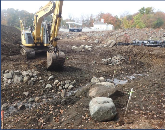
(left) Prior to the project, Toms Brook flowed between the two silt fences at the upper right corner, toward the gas station, behind the excavator and to the left of the camera. The new channel cuts the corner and will be located where the orange-flagged stakes are located.
