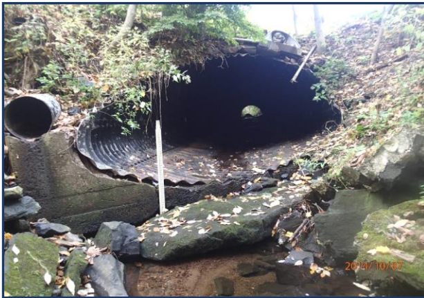
(left – before modifications) The Terry Brook Culvert outlet, perched over 2 ft. in height above the brook, blocked upstream fish passage
