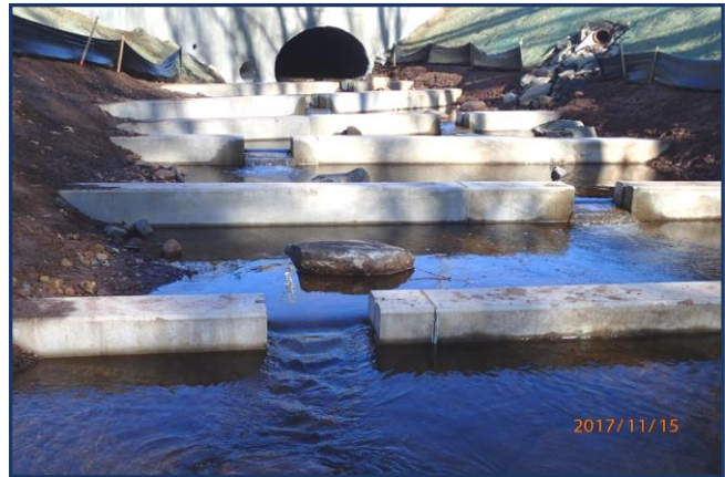
(right – after modifications) Upstream view of notched concrete weirs installed at outlet to provide upstream fish passage. Natural stream habitats were restored between the weirs.
